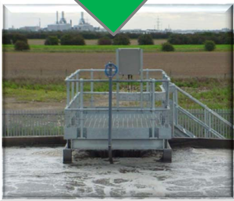
Platform over aeration process
