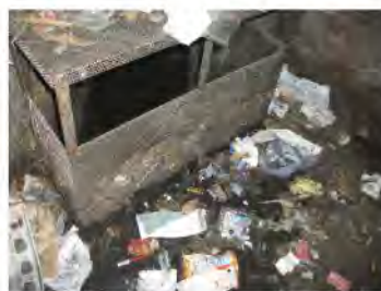
Connector Pipe Screen Keeps Debris in Catch Basin
