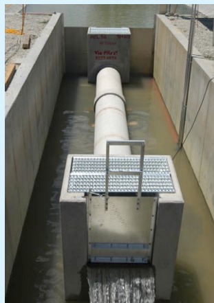
Figure 3: “Unearthed” Murrumbidgee Irrigation meter outlet showing the head/discharge drop boxes (sumps) with the resultant fully submerged pipe.
