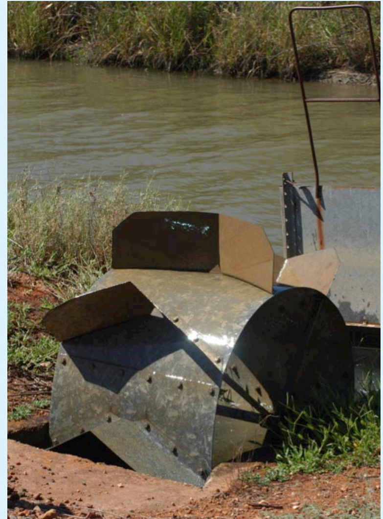
Figure 1: Dethridge wheel, note the large sharp vanes
