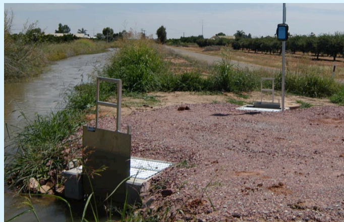
Figure 4: A completed MACE AgriFlo meter outlet. Head ditch is to left of photo.
